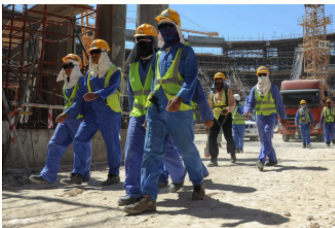
Even as far back as 2015, concerns over existing laws for migrant workers made headlines as Qatar won the bid unexpectedly. Pictured: Foreign workers in a Qatar construction site for the 2022 World Cup Stadium. Source: New York Times
